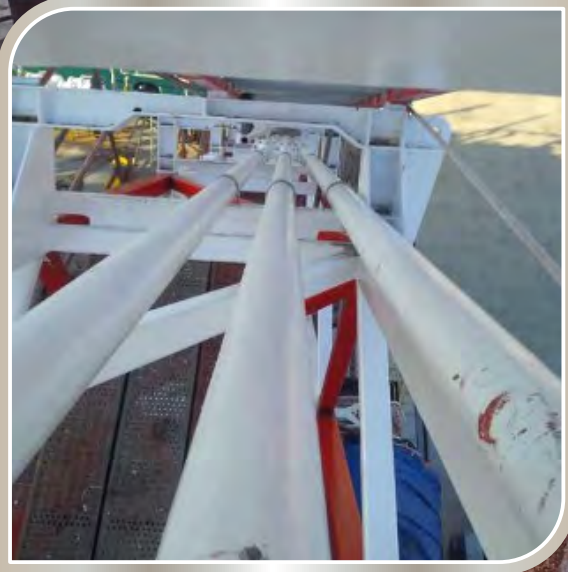
Flare Boom ( Fire Burner ) Lines Workings
